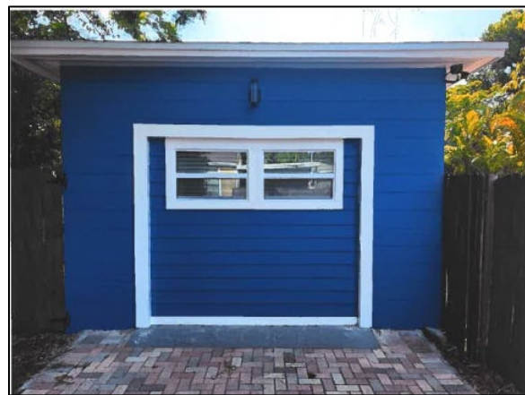
Figure 3: Hardi-Board siding and vinyl sash windows installed as part of garage enclosure (applicant photo)
